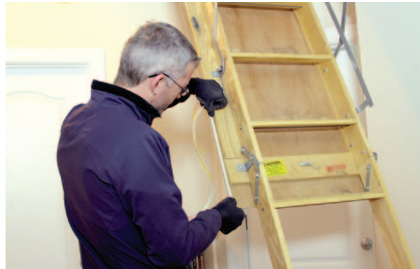
This standard attic hatch has been insulated and weather stripped to reduce energy waste. Photograph provided by EnergySmart Academy
